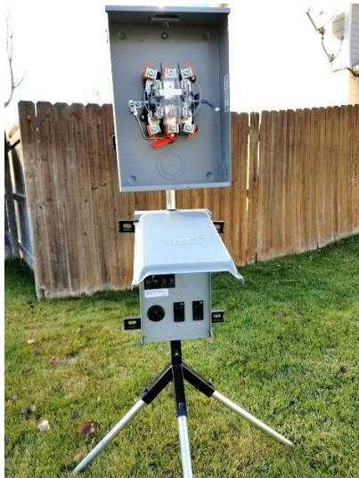
Stands for Temp Power
