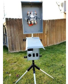
Stands for Temp Power
